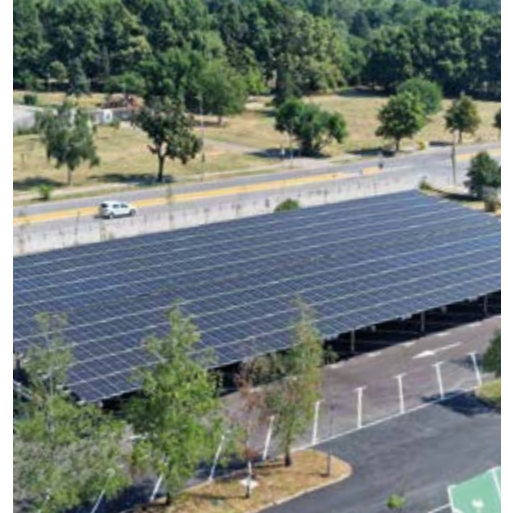
UNWE Photovoltaic Installations. Credits: UNWE
