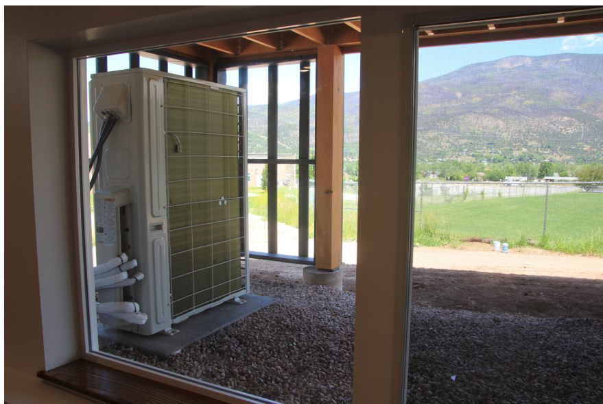
Figure 4.2.13. Air source heat pump (Best, 2020).
